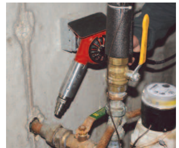
Heat pipes and more
